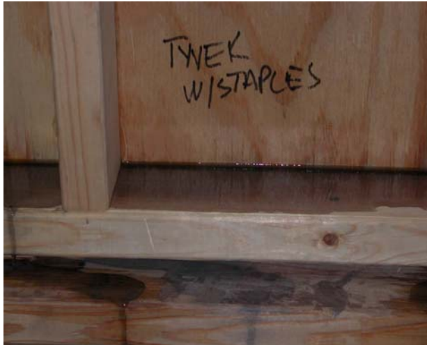
Figure 14. Water leakage in “Building Wrap A” panel during ASTM E 331 water spray testing.
