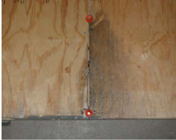
Figure 16. Indication of water leakage around cap fasteners in “Building Wrap A” specimen.
