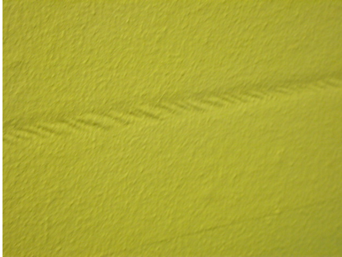
Figure 6. Wrinkles in joint treatment due to racking load. Joint treatment is StoGuard™ Fabric. Racking displacement is greater than 3/4-inch (19 mm) when photo was taken.
